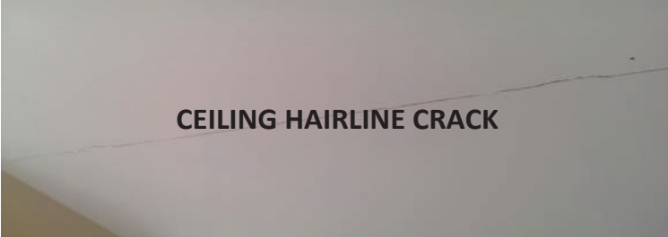
WINDOW & DOOR FRAME HAIRLINE CRACK
